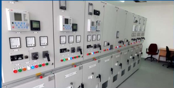
The switching station in Noordhoek received an upgrade of R4 million
