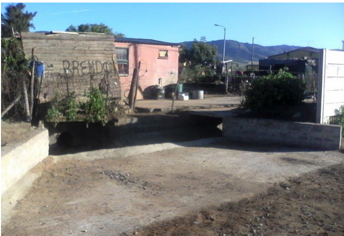
Storm water channel automatic overflow
