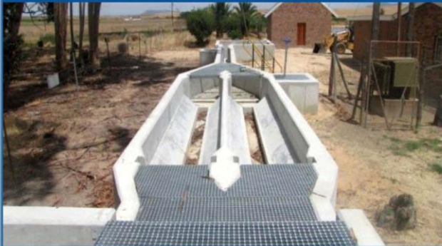
Waste Water Treatment Works in Porterville upgraded to the value of R25,6 million
