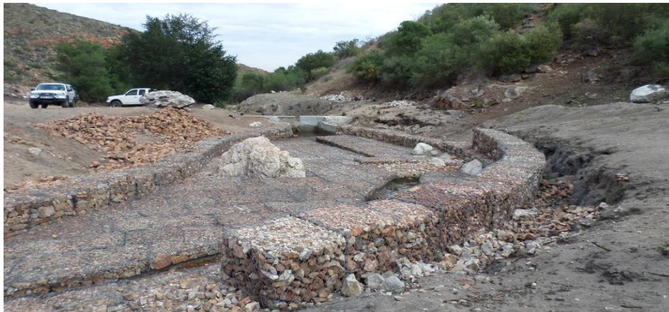
Inlet works Wittewater
