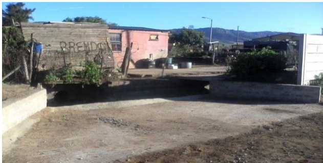
Stormwater channel automatic overflow
